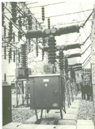
Figure 2. 132kV vacuum circuit breaker designed in the 1960's, in service in the UK.
