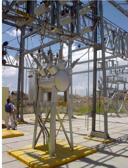
Figure 1 Modern stainless steel 38kV outdoor circuit breaker design in service in Mexico.
